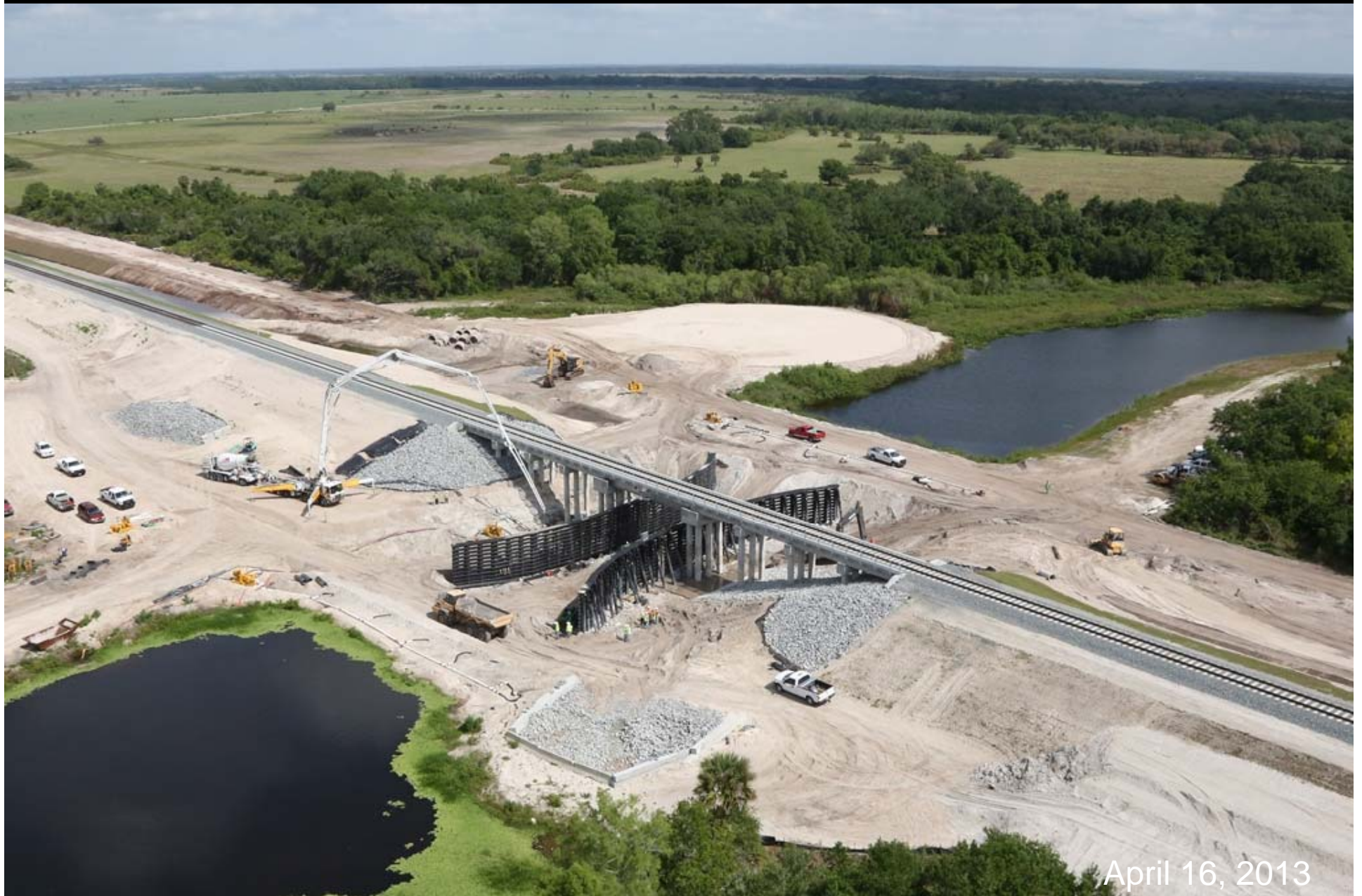
Railroad bridge construction is nearing completion in the Kissimmee River Phase II/III restoration area.
