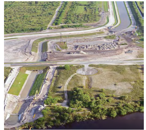
Florida expedites construction: The C-44 Reservoir and Stormwater Treatment Area project in Martin County will provide 50,600 acre-feet of storage to capture and treat local basin runoff to protect the St. Lucie Estuary.
