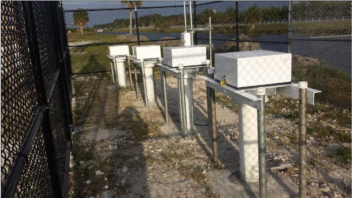
Figure 8. Close-up photograph of site with telemetry equipment installed.
