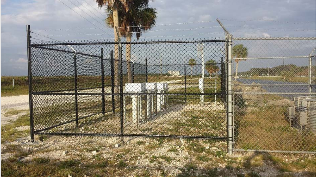
Figure 7. Site with telemetry equipment installed.
