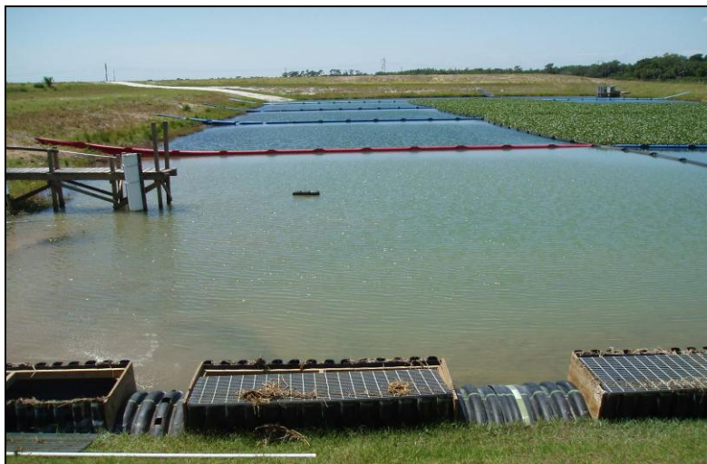
Figure 5-12. The Nubbin Slough HWTT facility. The mixing chamber and inflow manifold are in the foreground, and the outflow riser is in the upper right of the photo.
