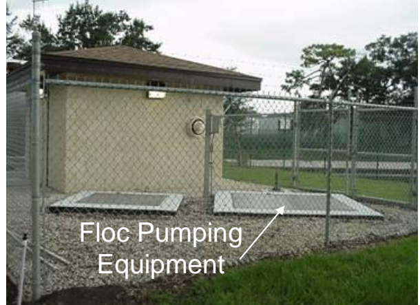
Floc Disposal System
