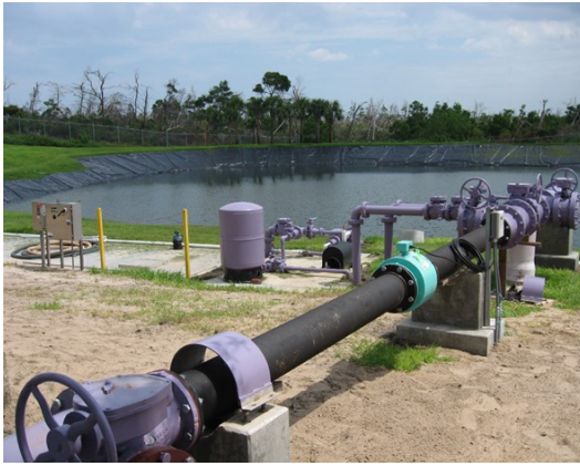
Reclaimed Storage Pond and Pump Station
