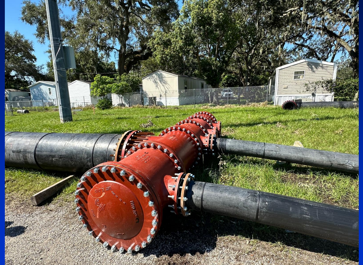
Manifold for 12" Mobile Pumps
