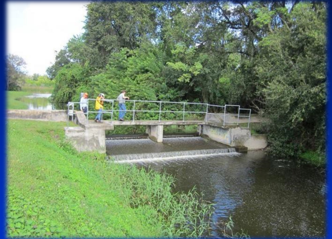
Lake Mare Prairie Control Structure
