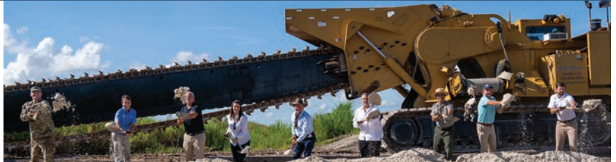
Groundbreaking for the CEPP New Water Seepage Barrier Wall on Aug. 20, 2021. L-R: Former USACE - Jacksonville District Lt. Col. Todd Polk, SFWMD Director Drew Bartlett, Congressman Carlos Gimenez, Lt. Governor Jeanette Nuñez, SFWMD Board Member "Alligator Ron" Bergeron, City of Sweetwater Mayor Jose "Pepe" Diaz, Superintendent of Everglades and Dry Tortugas National Parks Pedro Ramos, Everglades Foundation CEO Eric Eikenberg and Former DEP Southeast District Director Jason Andreotta.
