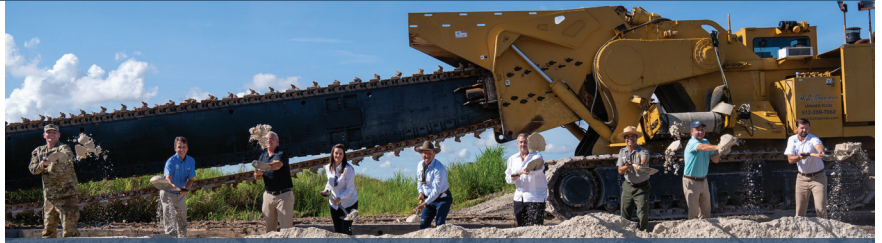
Groundbreaking for the CEPP New Water Seepage Barrier Wall on Aug. 20, 2021. L-R: Former USACE - Jacksonville District Lt. Col. Todd Polk, SFWMD Director Drew Bartlett, Congressman Carlos Gimenez, Lt. Governor Jeanette Nuñez, SFWMD Board Member "Alligator Ron" Bergeron, City of Sweetwater Mayor Jose "Pepe" Diaz, Superintendent of Everglades and Dry Tortugas National Parks Pedro Ramos, Everglades Foundation CEO Eric Eikenberg and Former DEP Southeast District Director Jason Andreotta.
