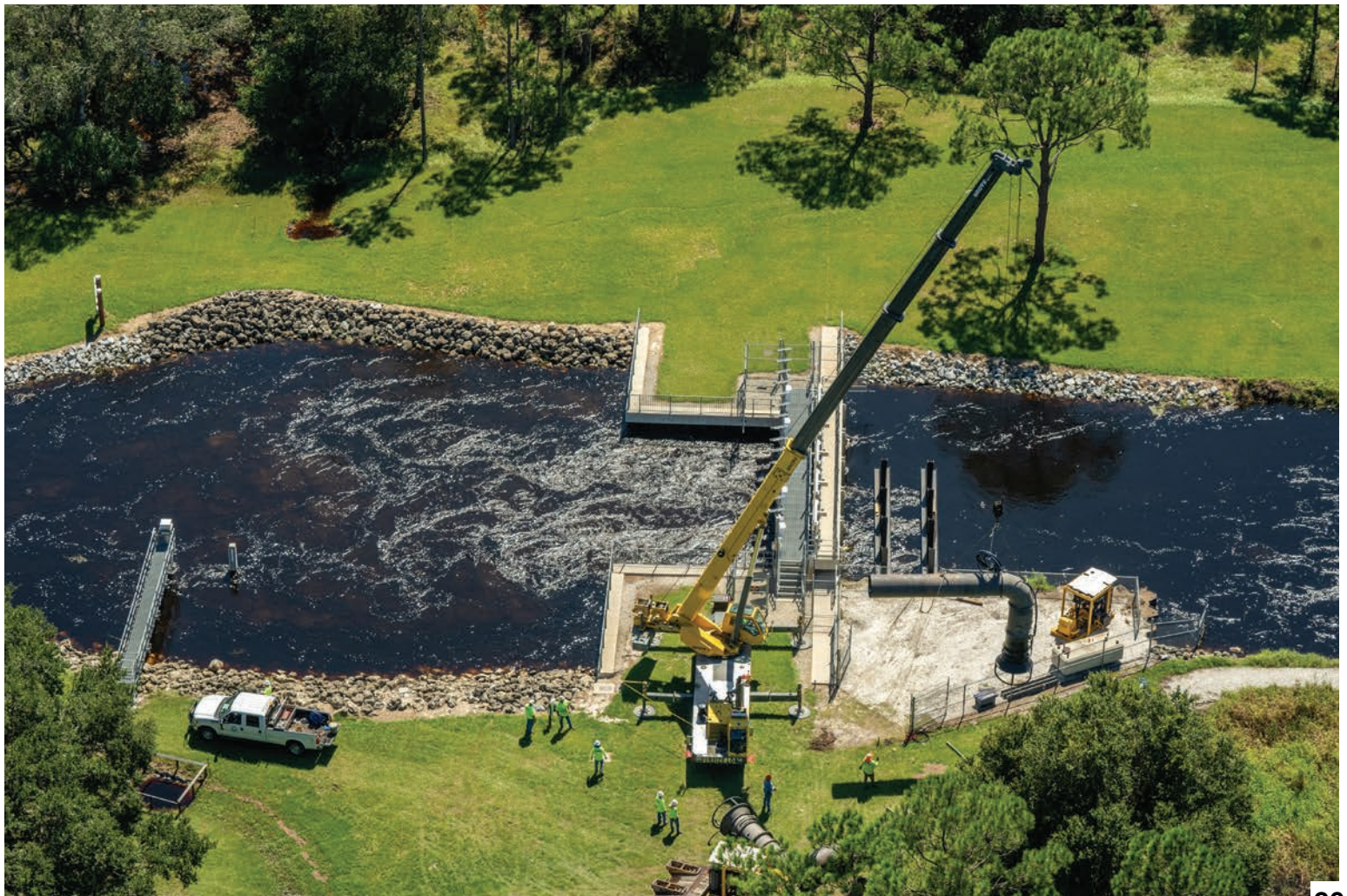
G-103 Structure after Hurricane Ian
