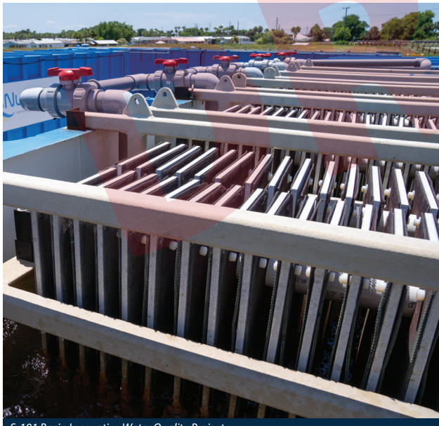
S-191 Basin Innovative Water Quality Project
