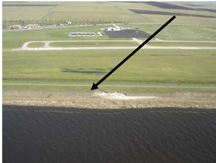
Figure 46. Lake Okeechobee levee damage from Hurricane Wilma (photo by SFWMD).
