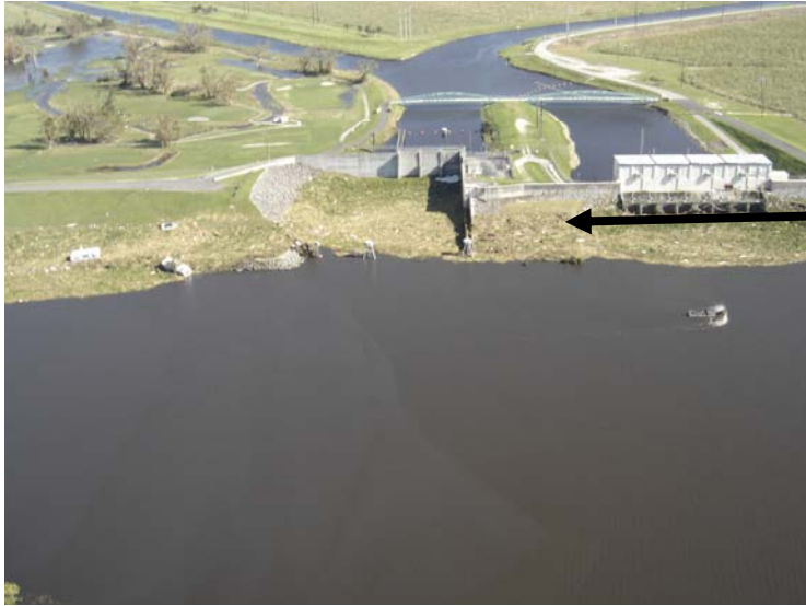
Figure 45. Vegetation pushed into hurricane gate S-351 and pump station S-2 along the south shore of Lake Okeechobee during Hurricane Wilma (photo by SFWMD.)
