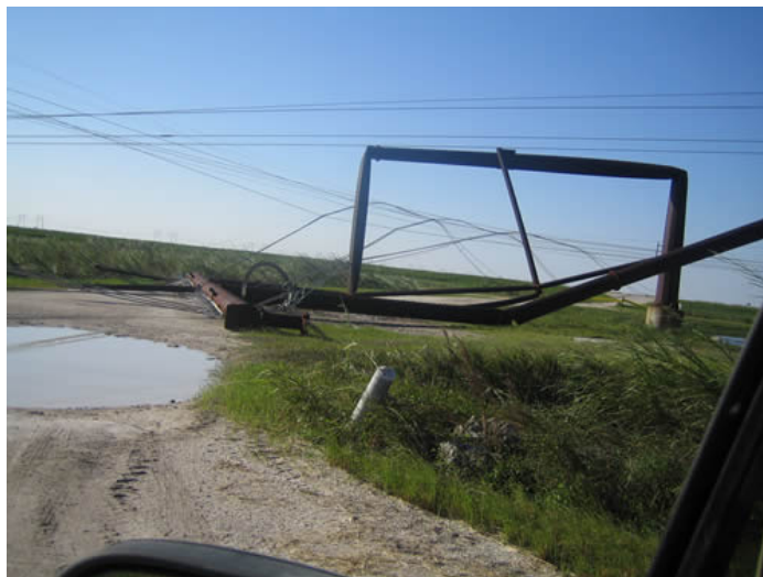
Figure 36. High-power transmission line damage by Hurricane Wilma in an STA (photo by SFWMD).
