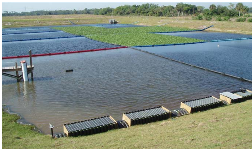
Figure 5-3. Nubbin Slough HWTT. The mixing chamber and inflow manifold are in the foreground and the outflow riser is at the upper right of site.
