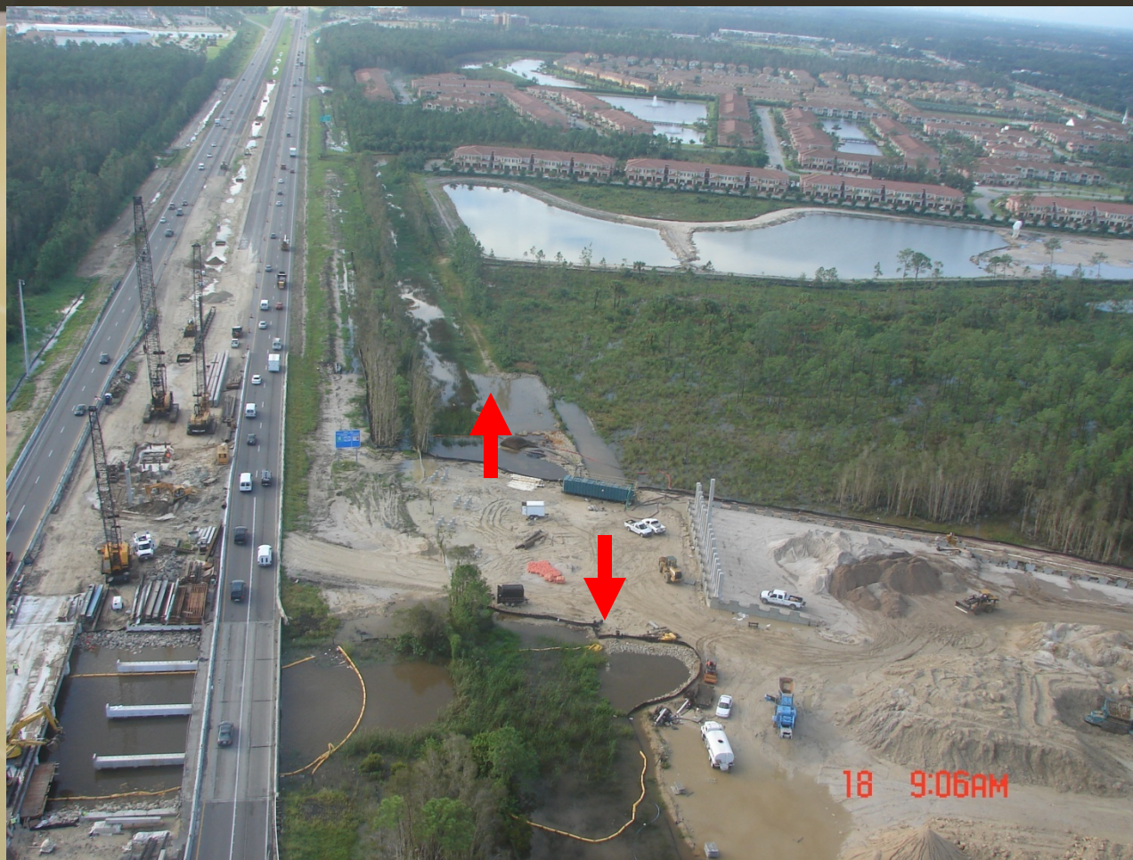
Construction Blocked Flow and Changed Flow Direction
