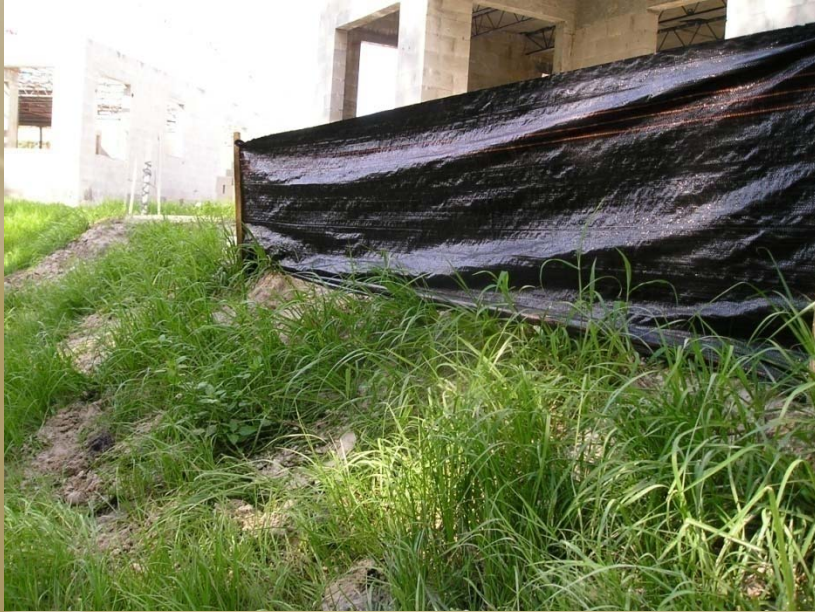
Silt fence not trenched
