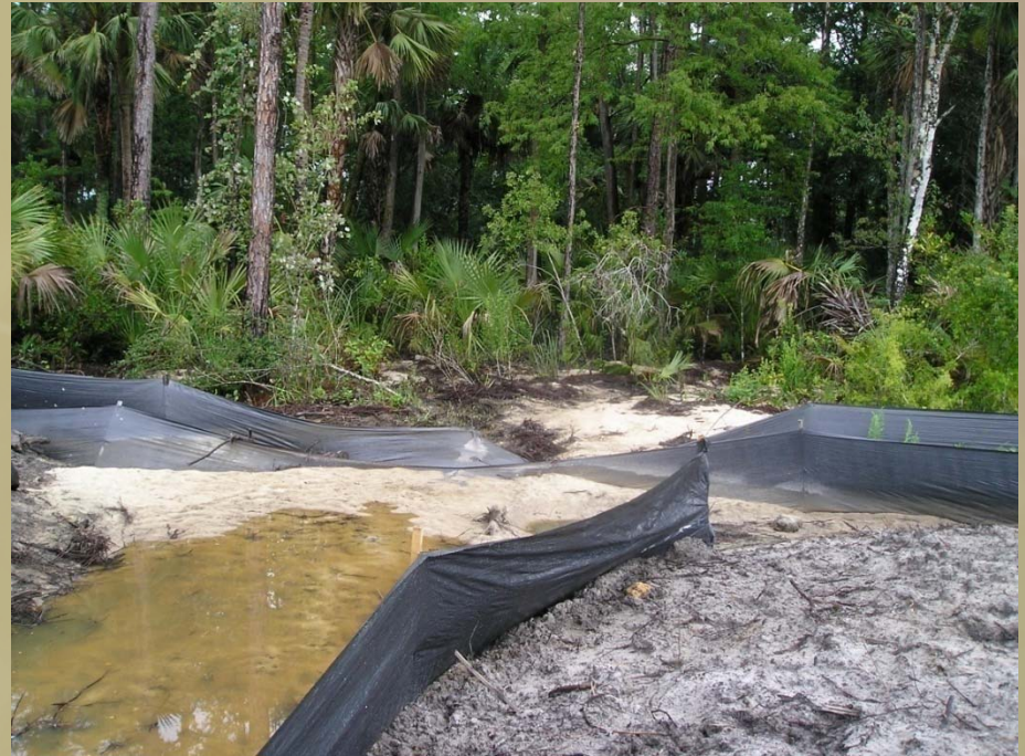
Silt fence breach
