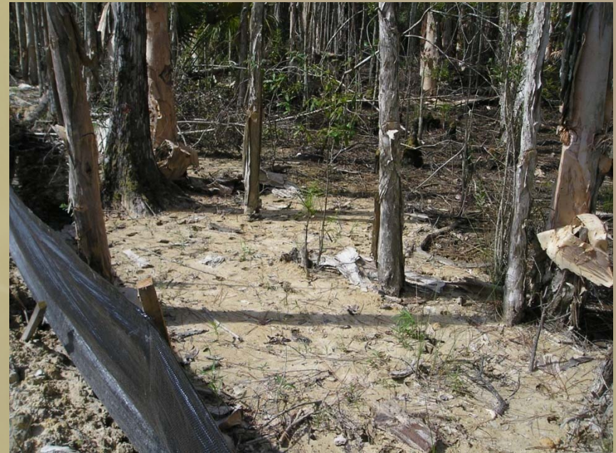
Silt fences not trenched
