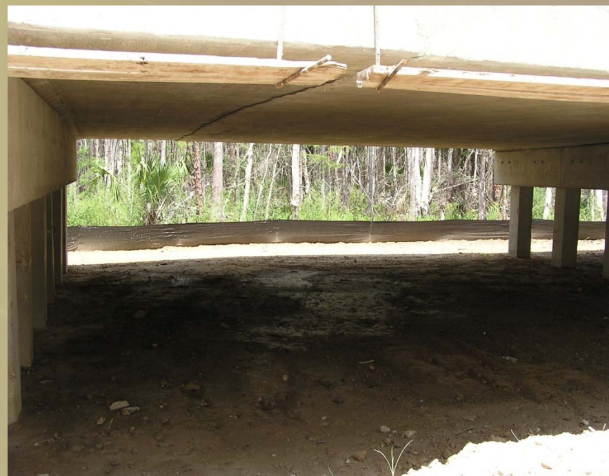
Silt fences installed properly but Flow-way blocked
