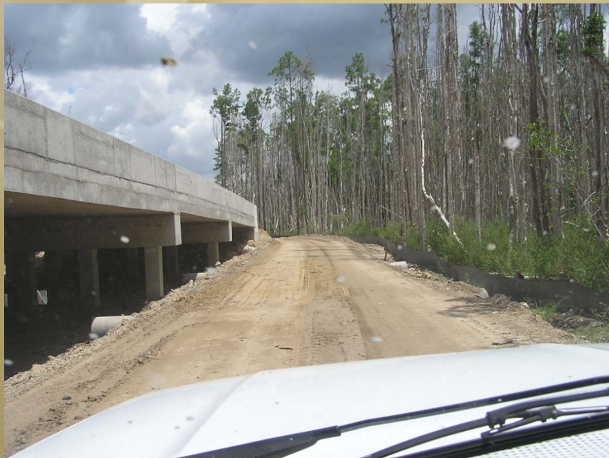
Construction road blocking Flow-way
