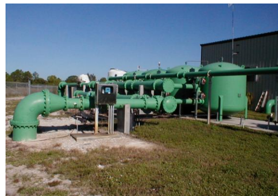
Part of Marco Island's ASR System
