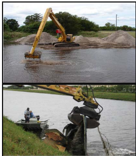
Crews remove shoal in Highlands County (top) and debris in Palm Beach County as part of efforts to keep canals clear and waterways running smoothly.
