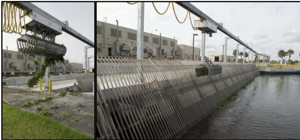
An automatic rake system in western Palm Beach County keeps a critical pump station clear of vegetation. (Click on the pictures for larger versions.)
