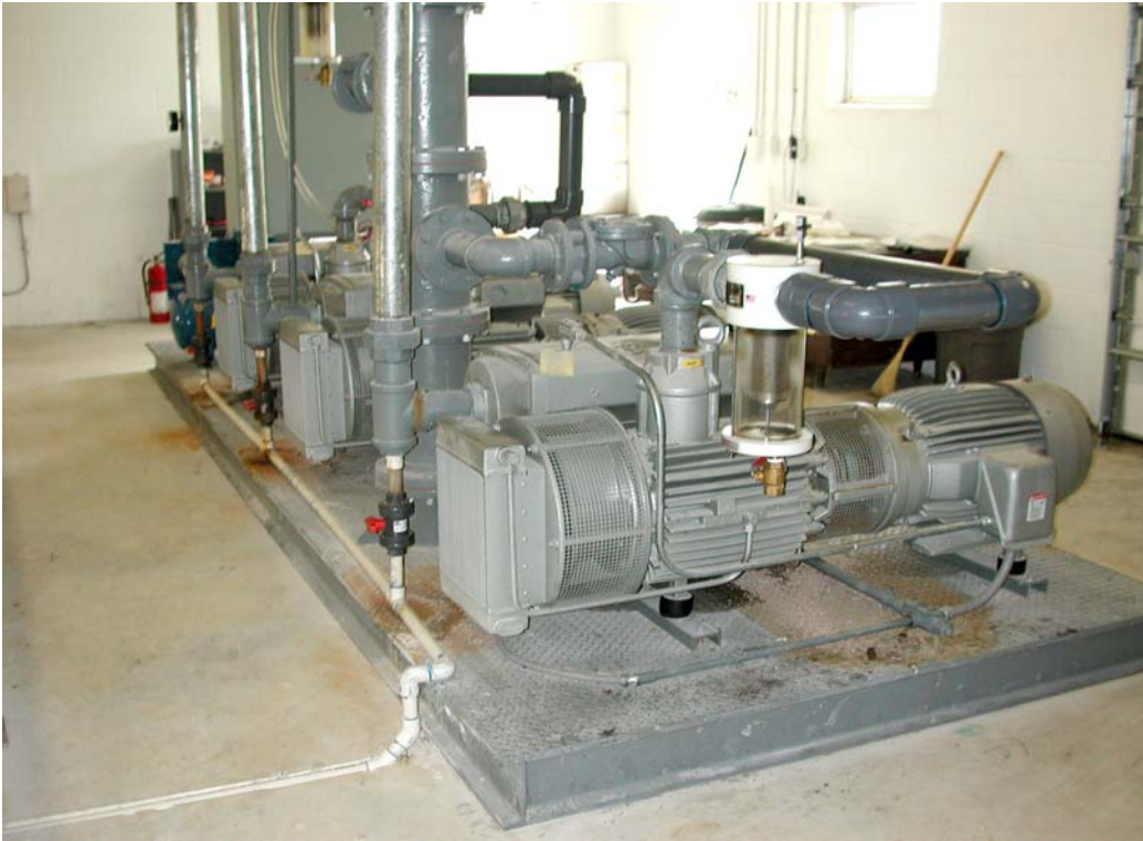
Vacuum System Pumps
